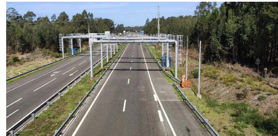
Tolling sensors on a Portuguese roadway
