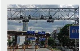
Tolling speed gantries in Bangkok, Thailand
