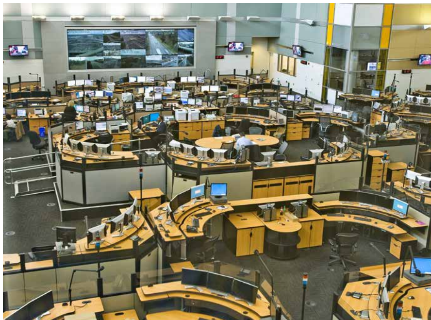
In Northern Virginia, Fairfax, the Virginia Department of Transportation operations centre is a US$125 million facility, manned by dispatchers with VDOT, the state police, Fairfax fire and rescue, and the Fairfax police
