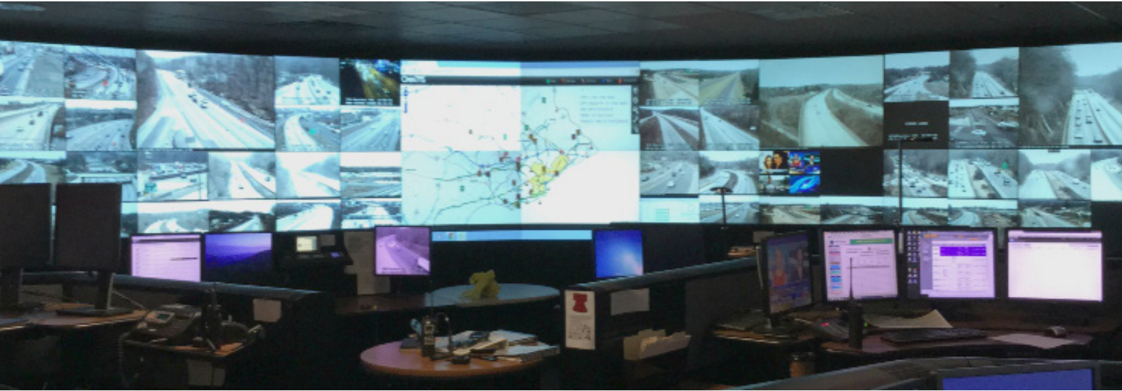
Traffic Management Center, Pennsylvania
