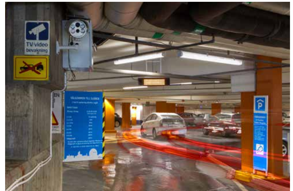
Car park management system, The Globe, Sweden
